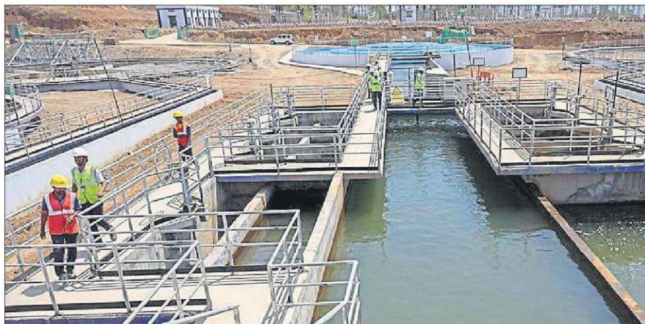
Water lifted from the intake is sent to reactor clarifiers after running it through a cascade aerator.
