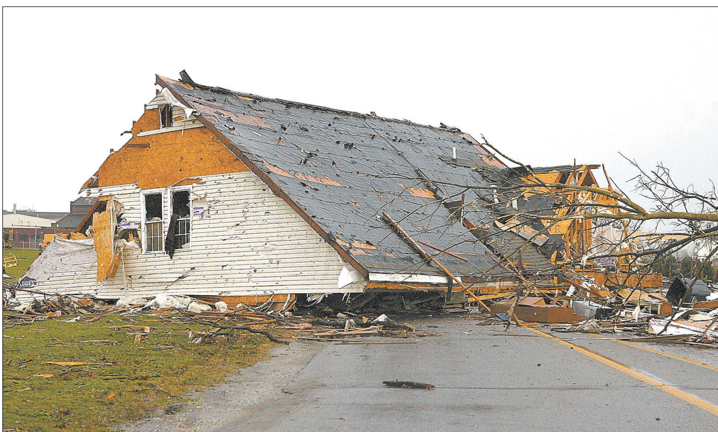
ICONIC IMAGE: The upper half of a home sits in the middle of Home Avenue near the intersection with Hoffer Street after the tornado ripped through Kokomo. Above, Phyllis Rawlins searches Monday through debris for items from her house that was destroyed on Ricketts Street.
