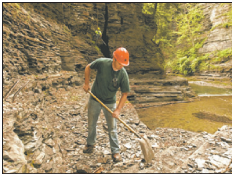
Marcus Whalen shovels rock loosened by the scaling crew as Alvin Walker, background, works up above the gorge trail in Robert H. Treman State Park. The gorge trail between the bottom of Lucifer Falls and the upper parking lot is closed until repairs can be completed. The rim trail is open. SIMON WHEELER / STAFF PHOTO
