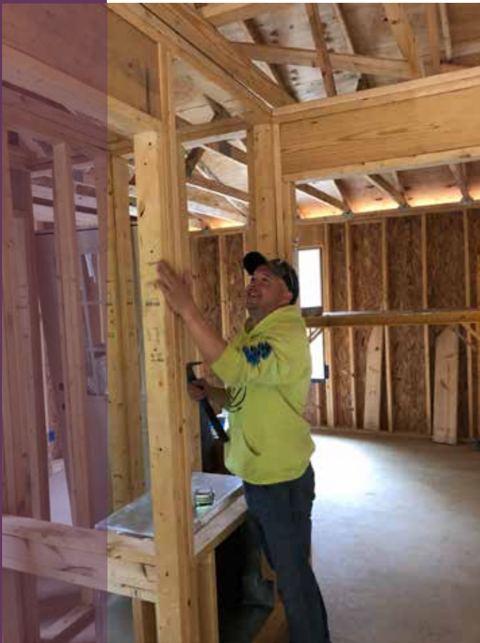
Tesdahl does electrical work in the Kentucky home the group helped build.
